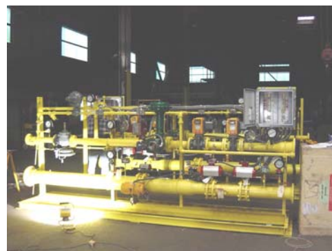
Coke oven gas & natural gas valve train
