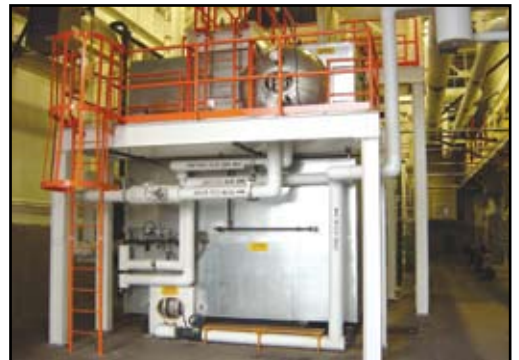
Boiler Blowdown System
