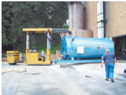
New Firetube Boiler during move-in
