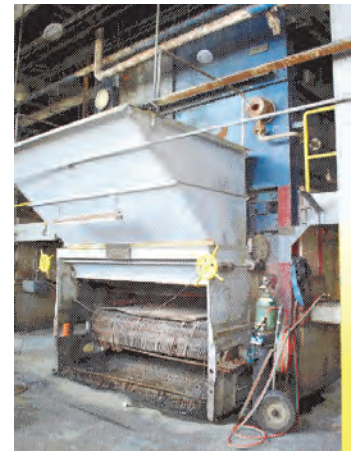
Coal Boiler prior to Demolition
