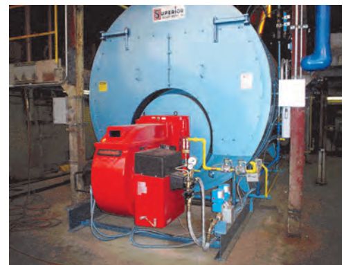
Installed Firetube Boiler w/Dual Fuel Burner
