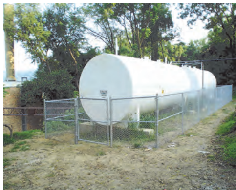
Installed Fuel Oil Storage Tanks
