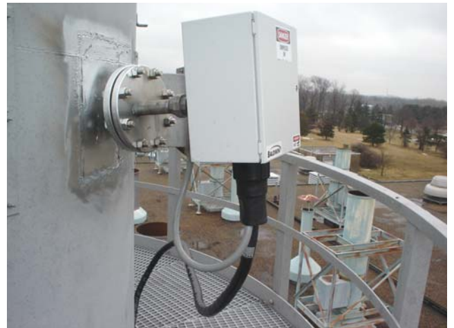
Flue gas probe on stack
