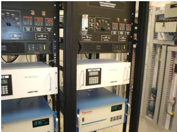
Rack mounted analyzers
