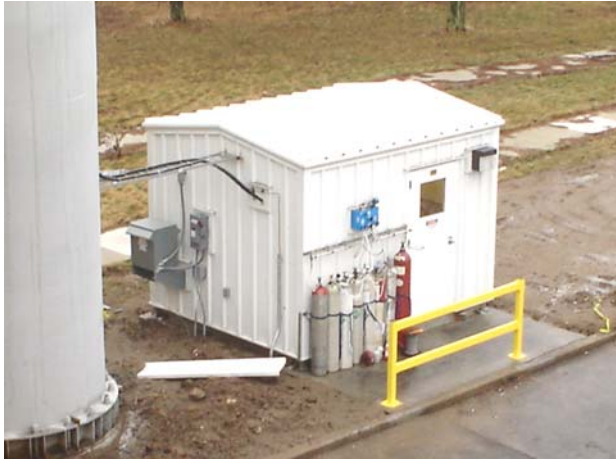
New CEMS equipment enclosure
