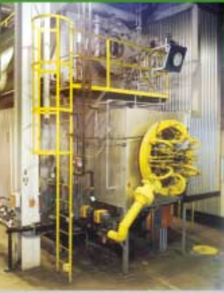
Low-NOx burner upgrade for an automotive assembly plant.
